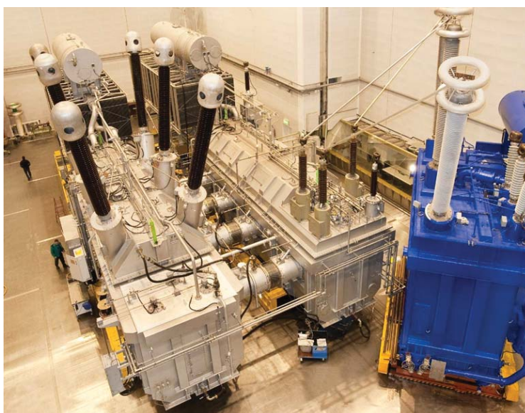
Obr. 9: Transformátor PST - S_n = 600 MVA, U_n = 400/400 kV, \alpha = \pm 40^\circ
