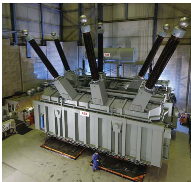
Obr. 8: Transformátor PST - S_n = 1400 MVA, U_n = 400/400 kV, \alpha = \pm 25^\circ
